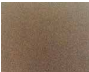
rust- epoxy fine texture
